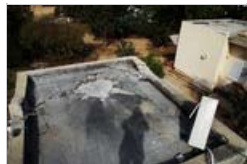
Click photo to download. Caption: The damage from a direct hit by a Gaza rocket on an Eshkol Regional Council "safe room" Nov. 16. Credit: Ronit Minaker.
